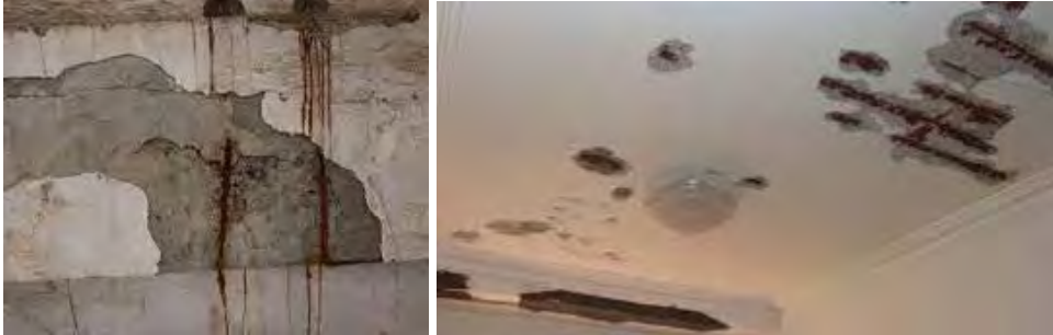
Figure 7-2: Corrosion of steel due to concrete spalling
