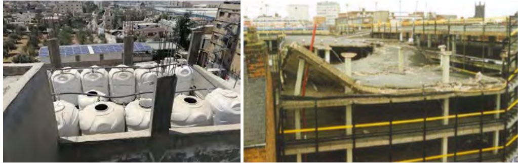
Figure 7-5: Overloading of roof slabs and failure possibility
